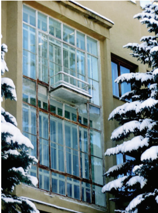
Fig. 38 Western Façade of Eastern Wing. Glass Curtain Wall and “Suspended” Balcony. (Photo Udovicki)
